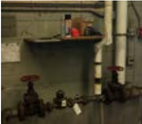
Original boilers, tanks and pipes, circa 1957
